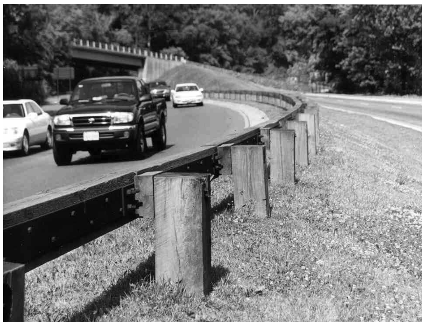
Figure 5-18. Backed Timber Guardrail
