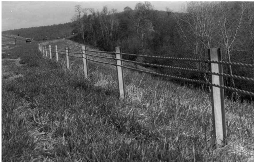
Figure 5-5. Three-Strand Cable Barrier
